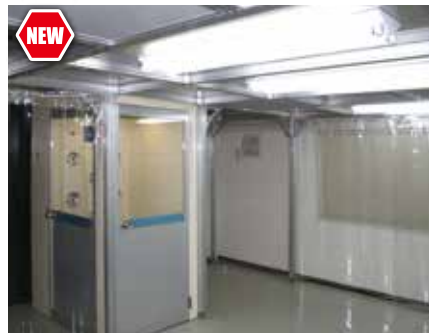
Large clean booth / air shower
